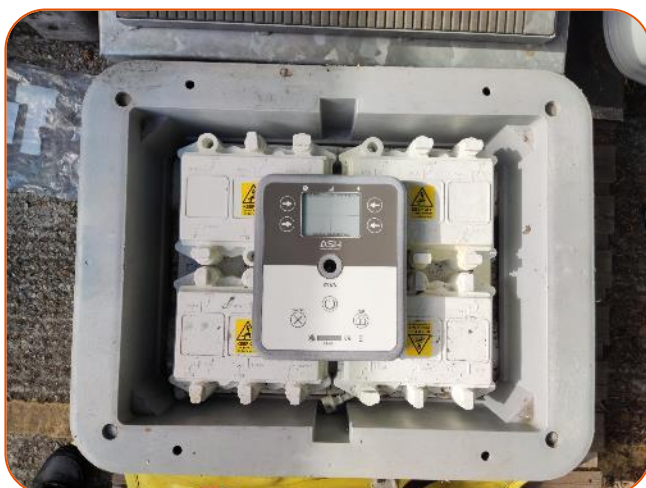
4-way Link Box Switch
